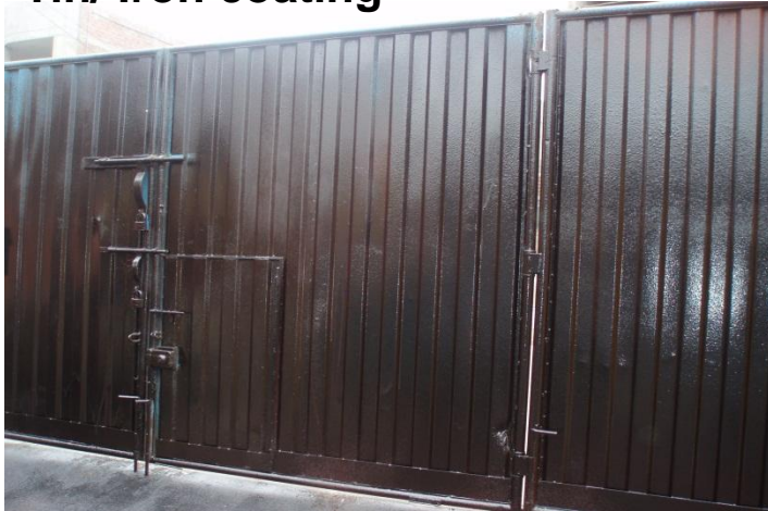
Tin/ Iron coating
